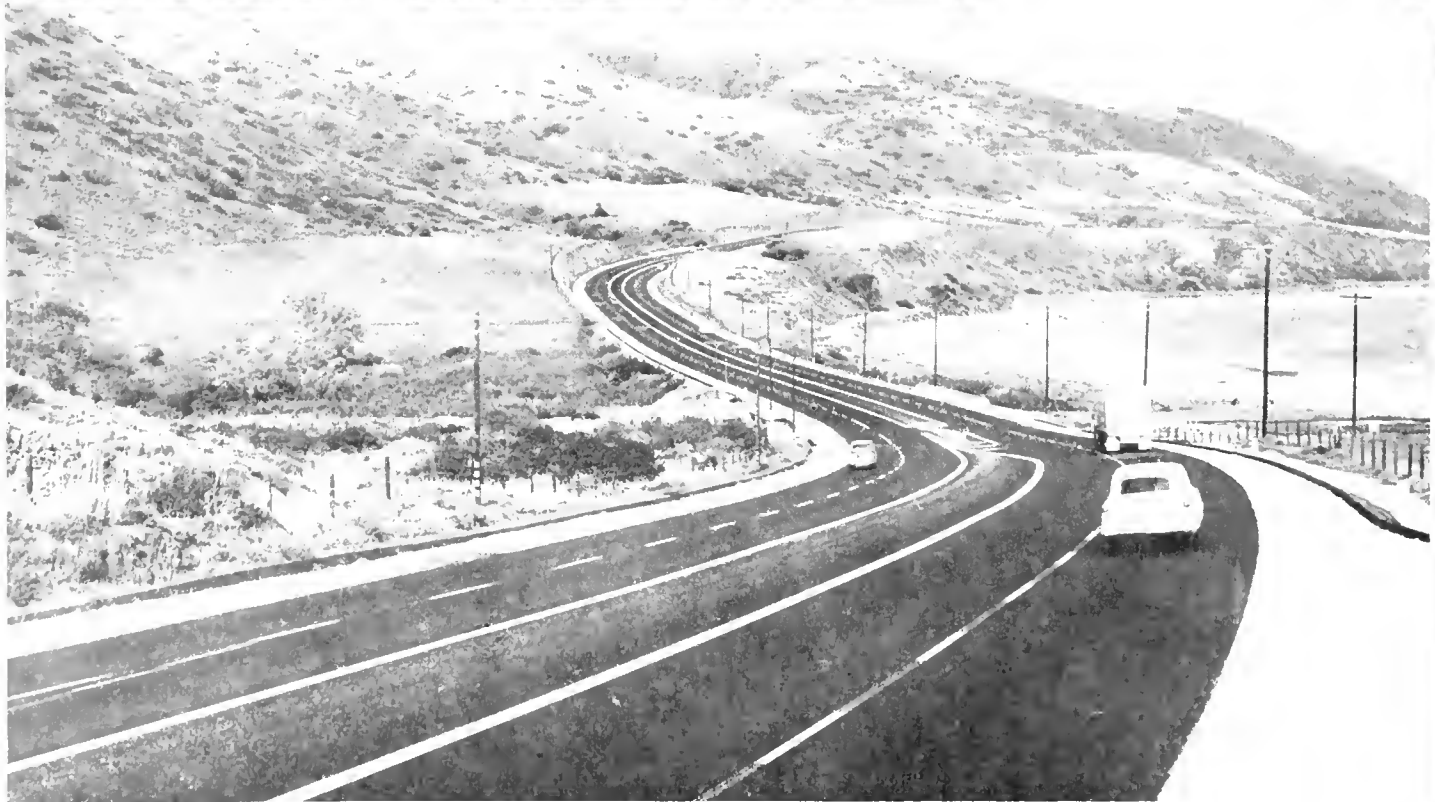
UPPER Looking easterly from Little Sycamore Canyon, showing in foreground channelization lane for Yerbo Buena Road. This section of the project is in Ventura County, with Los Angeles county line just beyond limits of photograph. At left, grading operations are in progress by abutting property owner under permit, to provide a location for a service station, business office and restaurant. LOWER Looking easterly along completed divided highway, showing in center the widened bridge across Arroyo Sequit Creek. Extending, center left, is Mulholland Drive, that goes up Arroyo Sequit Canyon. The striping has been carried out to provide left turn lane into Mulholland Drive.
